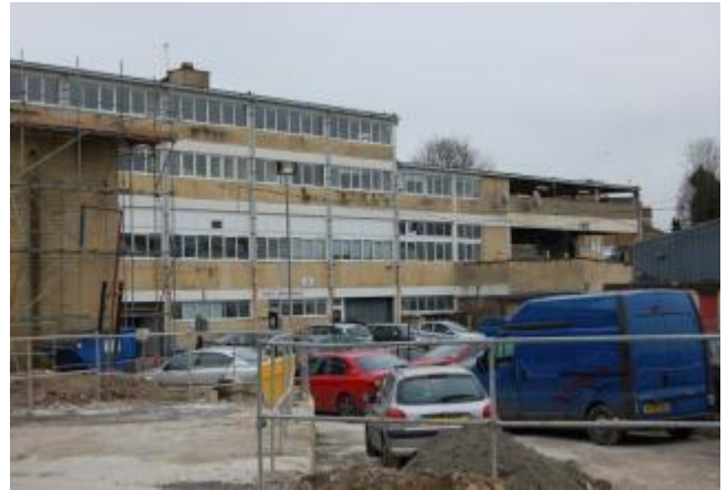
Photograph 8. View of building 1 from the rear showing the offices and undercover parking (RHS)
